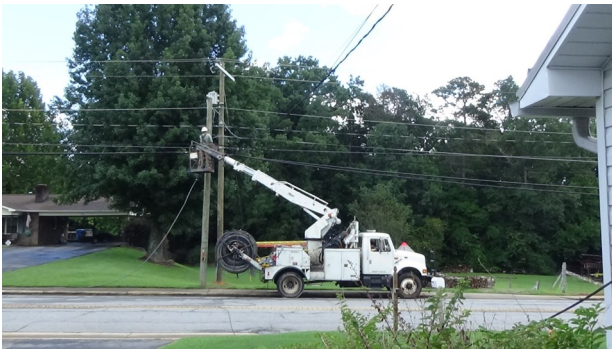
On August 19, a contractor connected a cable to a new pole erected earlier in the summer.
