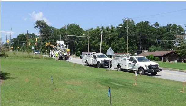
After Miller Pipeline left on August 26, electrical crews removed a utility pole no longer needed.
