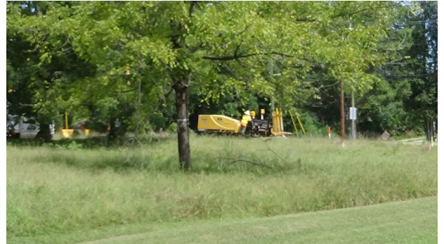
Miller Pipeline moved heavy equipment into place on the corner of Pinewood and N. Highland on September 6.
