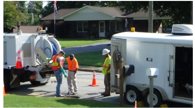
Employees of the Town of Granite Falls worked with employees of Miller Pipeline to check the sewer on August 26.
