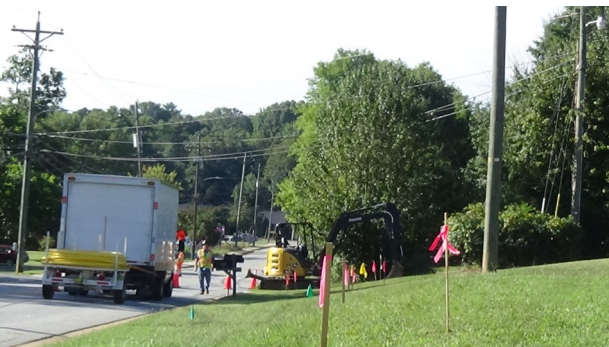
Miller Pipeline installed a yellow pipe that sticks up out of the ground on September 6.
