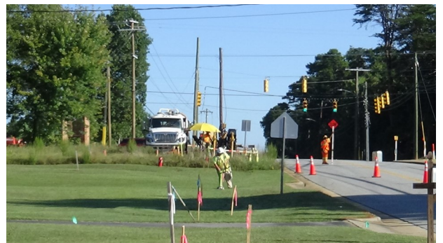
Someone from Miller Pipeline used special equipment to check along the route of the new pipeline on September 6.
